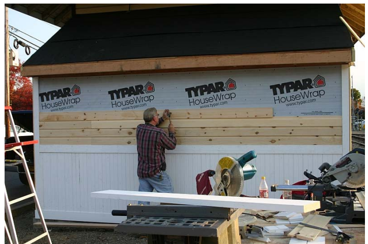
KC Smith puts up the siding for the new addition. The addition houses a larger storage closet and the stairwell to the new basement
