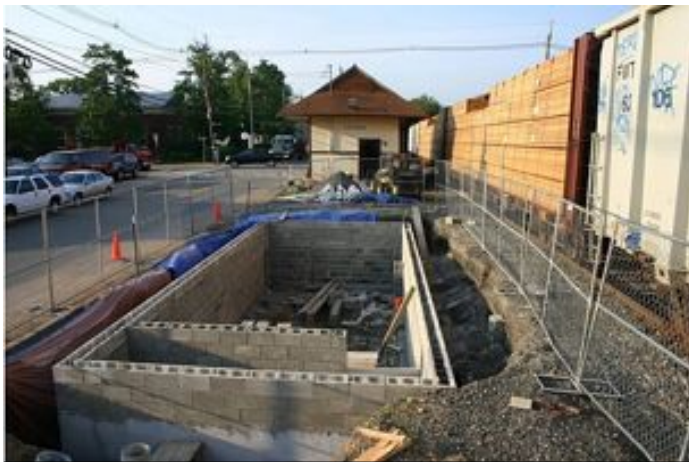
The new foundation gives the station a brand new feature – a basement.
