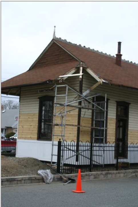
Now safe from the threat of countless trucks, the northeast corner of the station's roof undergoes repair for, hopefully, the last time.
