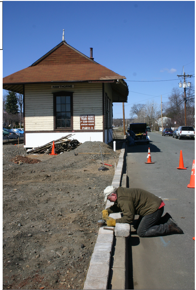
VRA President KC Smith works on the new curbing along Royal Avenue.
